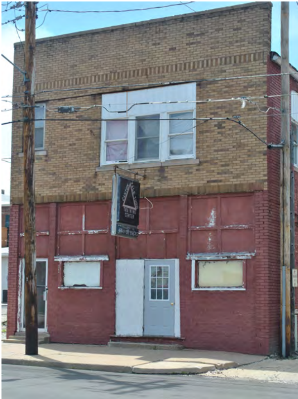
Figure 25: Deteriorating facades restricting sense of place
