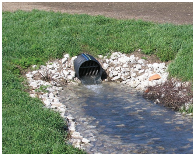
Fig. 7.2 Flowing tile drainage outlet (source: G. Czapar/UIUC)
